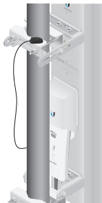
Placement on a Sector Antenna
